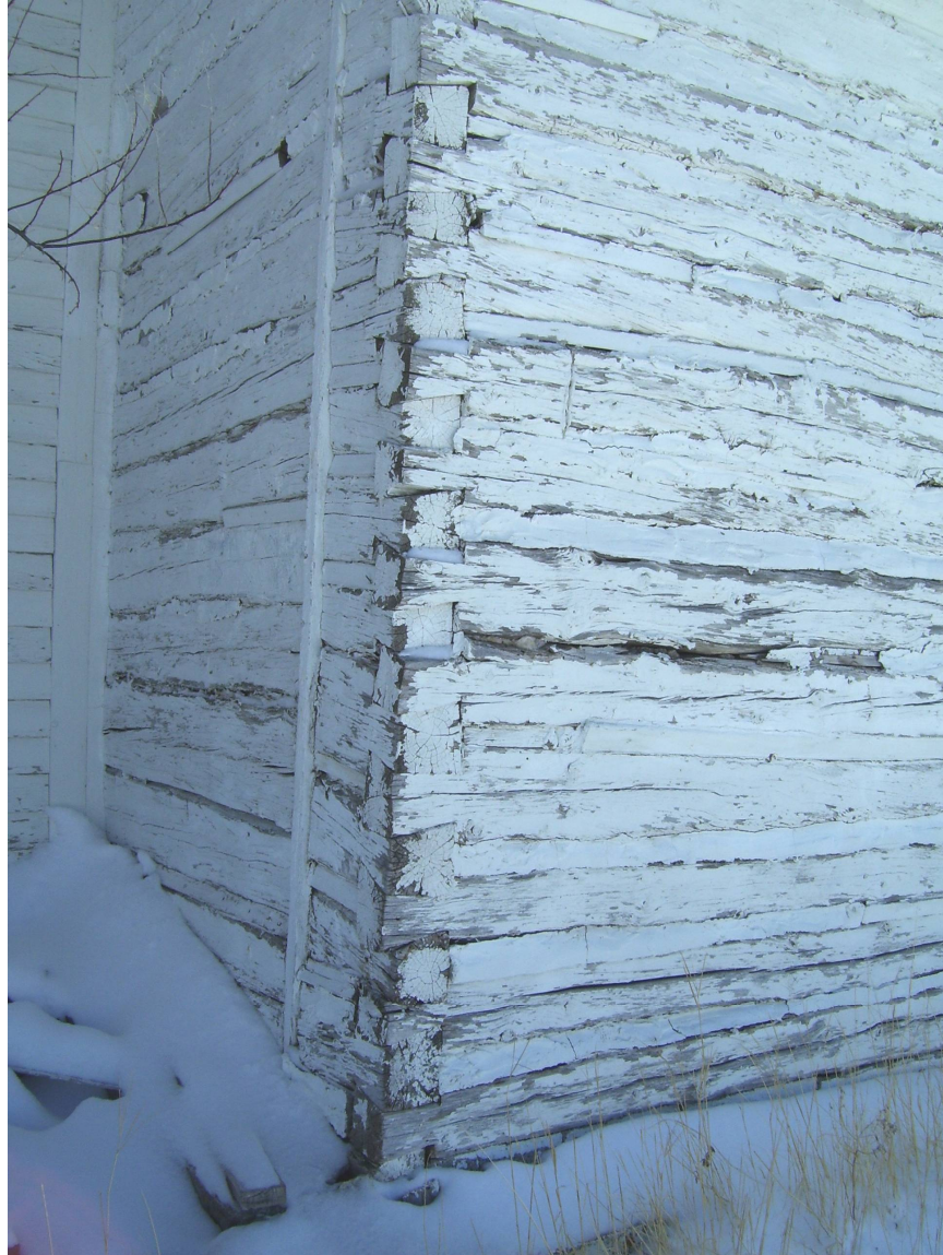
Detail of the log notching on the Church. Photo by L. Barkwell, 2009
